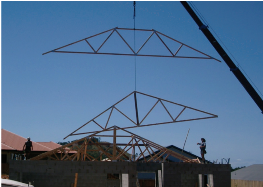
Photograph 3 – Incorrect lifting of trusses
