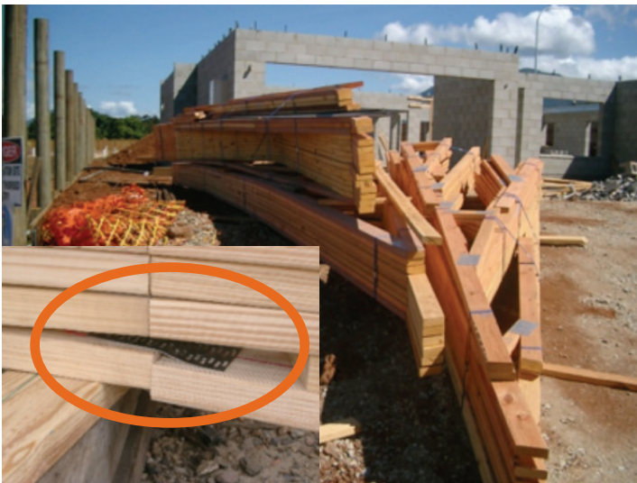
Photograph 1 – Don't install site damaged trusses or those with manufacturing faults. Replace or repair before erecting
