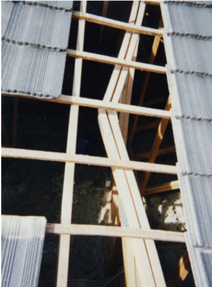
Photograph 5 – Inadequately fixed roof battens resulting in lateral buckling failure of girder truss
