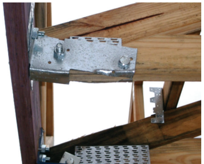
Photograph 7 – Girder brackets not installed correctly
