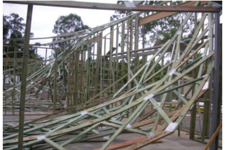
Photograph 4 – Dangers of not providing temporary bracing
