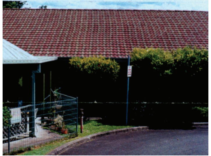
Photograph 6 – Distorted rows of roof tiles and trusses due to inadequate roof bracing
