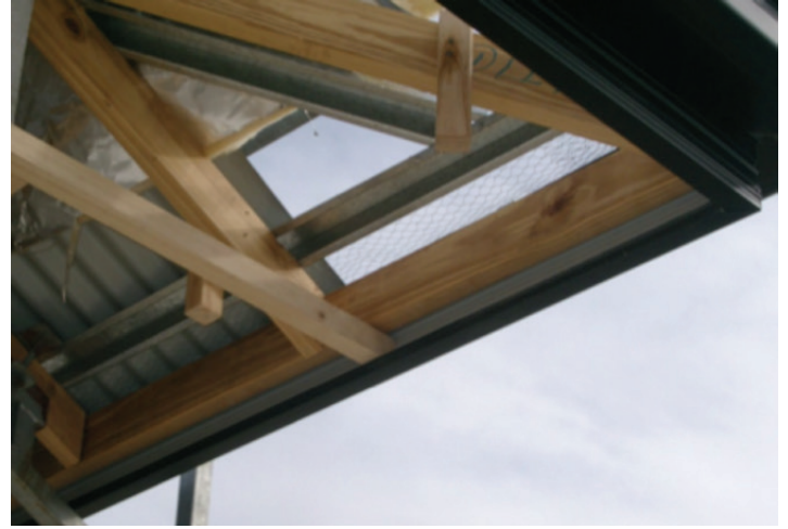
Photograph 9 – Ensure structural fascias are installed in accordance with the truss design and specifications
